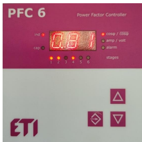
Figure 8. Reactive power compensator panel with the performed compensation results
