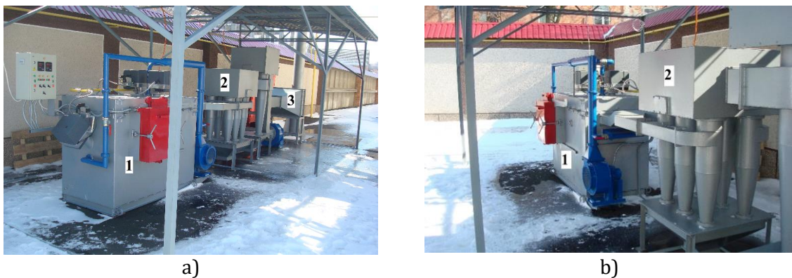
Figure 1: General view of the pyrolysis plant for the disposal of household waste a – view from the left; b - view from the right
