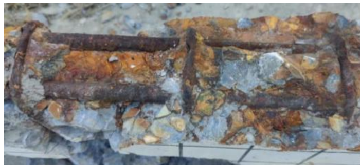
Figure 6. Corrosion of steel bars.
