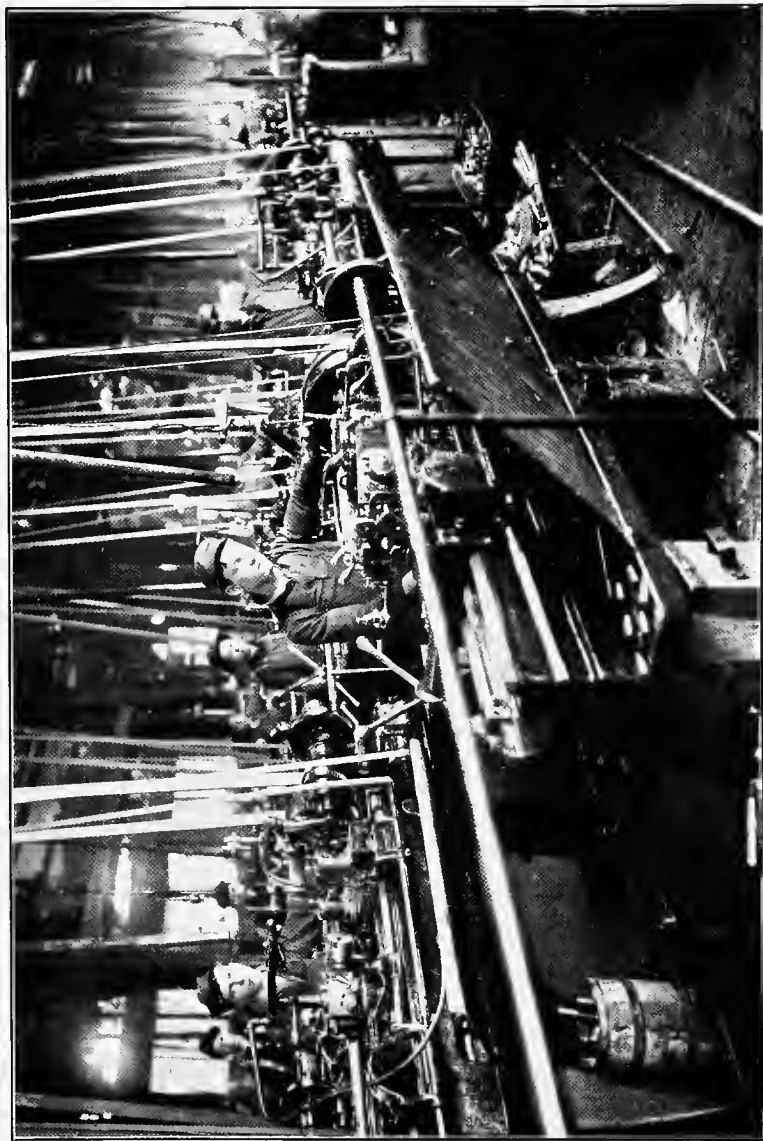
MACHINE ROOM SHOWING INTRICACY OF EQUIPMENT. GEARS GUARDED Courtesy Westinghouse Machine Company
