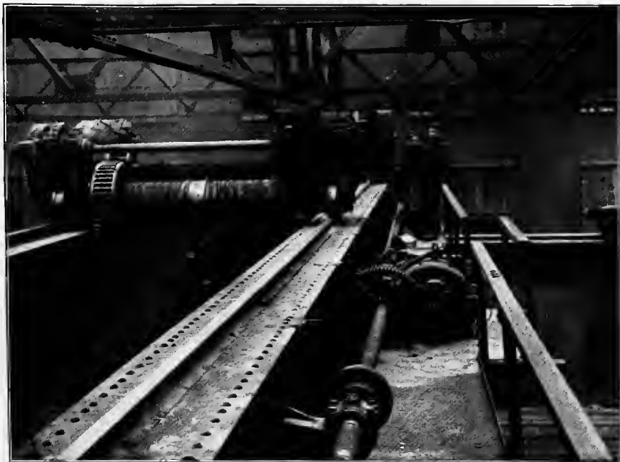
PLATE 7.—ELECTRIC TRAVELING CRANE BOUGHT ABOUT TEN YEARS AGO This shows open gearing, overhung gears, exposed couplings, etc.; the foot-walk on which the men are standing was placed on the crane after it had been installed
