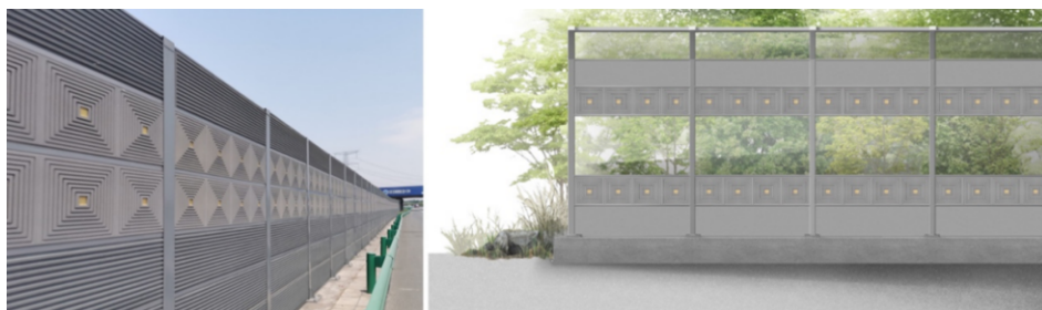
Figure.8 Jingyang Section of Xi'an North Ring Expressway Noise Barrier.
