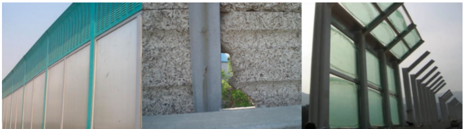
Figure 5. Current Situation of Noise barrier in China.
