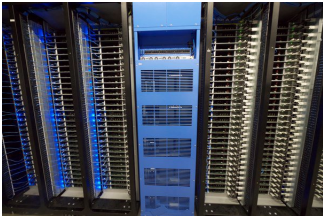
Figure 2: Picture of actual populated racks and battery cabinet. Racks are organized into triplets, each holding 90 servers and two 48-port switches. One battery cabinet provides backup power to the two triples pictured.
