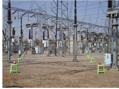
Fig. 3. A view of the 440 KV power distribution yard, showing the layout of equipment; apart from the transmission towers, several transformers and a firewall can be seen at a distance.
