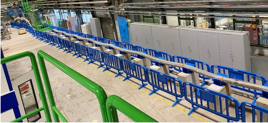
Fig. 4. View of a demonstration Cold Powering System – Demo 2 – tested at CERN for cryogenic and electrical qualification. The SC Link is 62.5 m long and it contains a full cross section \text{MgB}_2 cable assembly of the type needed for the powering of the HL-LHC Triplets.
