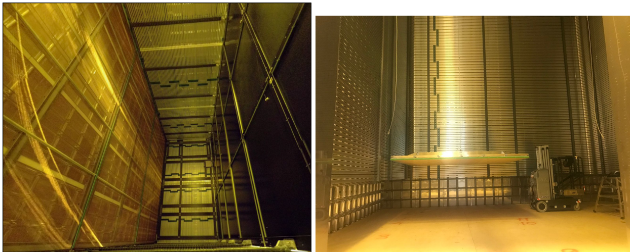
Figure 2: (left panel) Drift volume of the SP ProtoDUNE detector with an Anode Plane on the left and a Cathode Plane on the right; (right panel) first Charge Readout Plane being installed in the DP ProtoDUNE detector.
